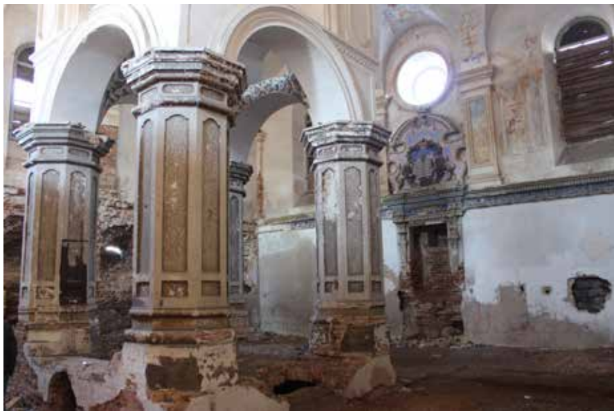
Interior of the synagogue in Slonim. Courtesy of the Foundation for Jewish Heritage
