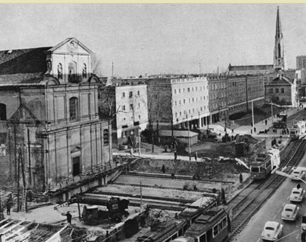
The Carmelite Church being moved in 1962 to permit widening of the street now called Aleja Solidarności.
